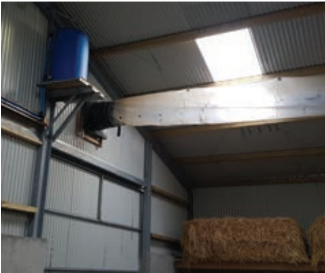
Figure 2: Positive pressure tube ventilation is the most used mechanical ventilation. Photo: Animal Health Ireland.
